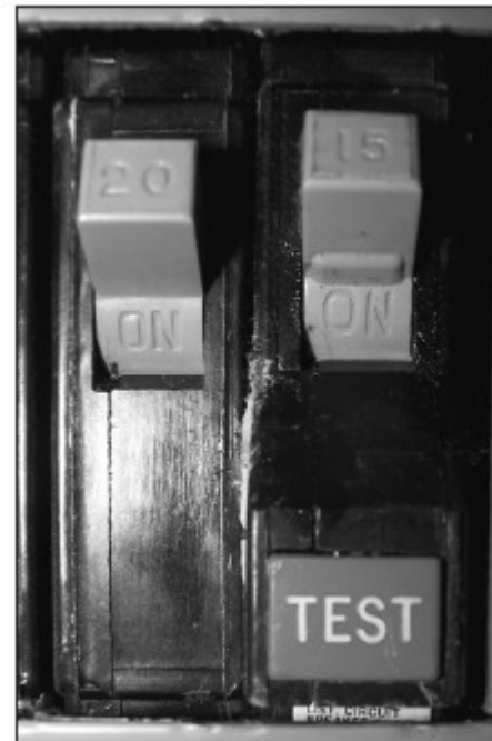
Ground Fault Circuit Interrupter (GFCI) circuit breaker
